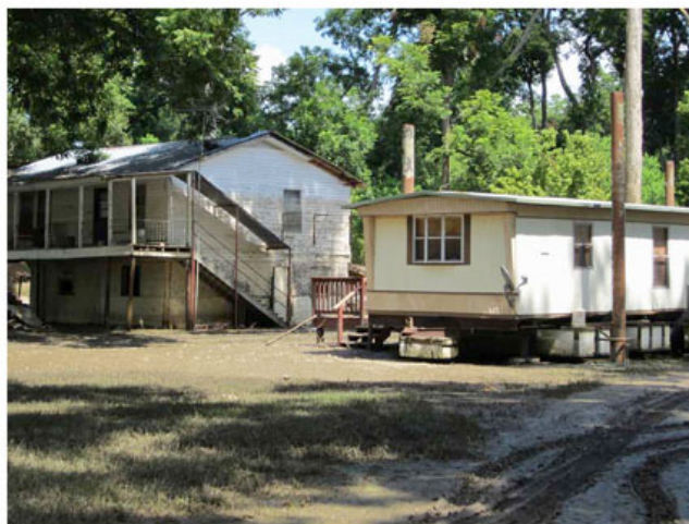
A 2011 Louisiana flood submerged the conventional house on the left almost to the rafters, as the high-water mark shows. Its neighbour, equipped with a homemade buoyant foundation, was undamaged. (Photo: Courtesy of Elizabeth English)
