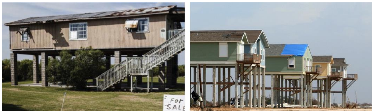
Fig. 1 Statically elevated houses on the Gulf Coast with extensive roof damage (William Widmer; FEMA/ Greg Henshall)
